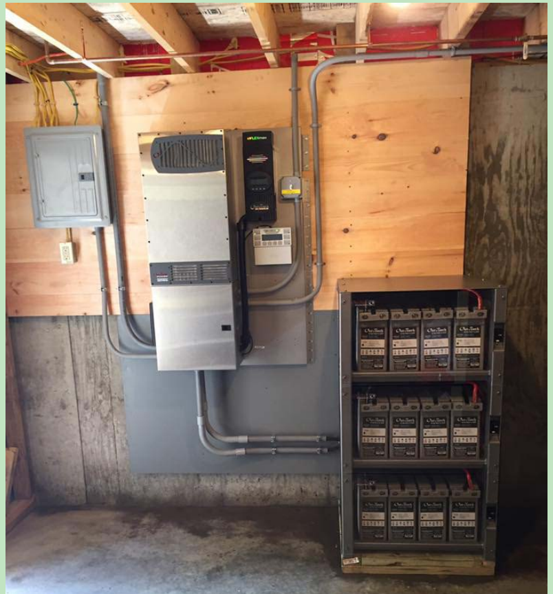
Battery bank and circuitry.
